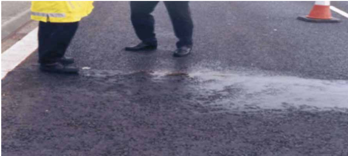
Figure 8.4.4 - Water ponded on surfacing at interface between a negatively textured thin surfacing and dense surfacing
